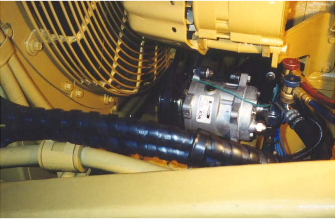
Compressor showing set-up and hose routing.
