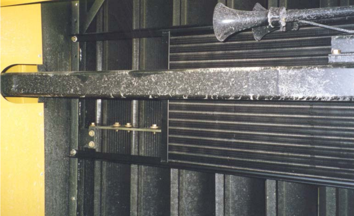
Left side of condenser as viewed from in front of the truck.
